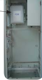
19" Active Equipment Section
